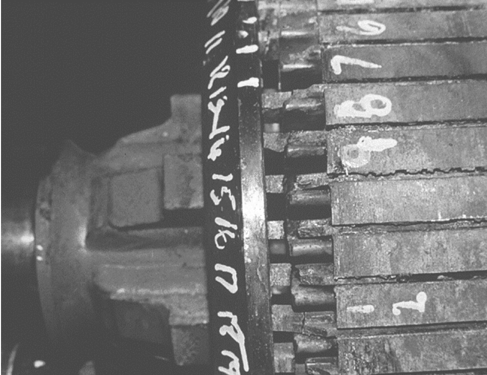
Figure 6-5. View of the motor rotor shows severe damage where rotor bars are broken away from the end ring.
